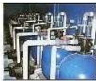
Fish Hatchery Filtration
