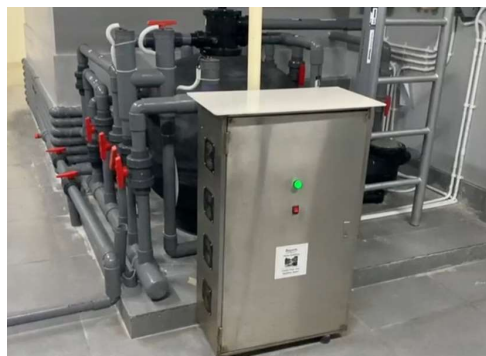
Figure 5, Water treatment installation at the apartment in menteng, jakarta.
